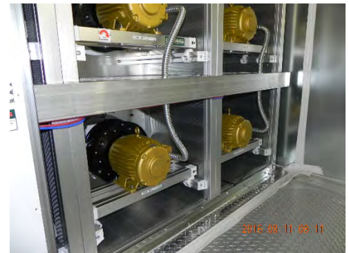
Figure 1: Multiple fans comprise the fan wall
