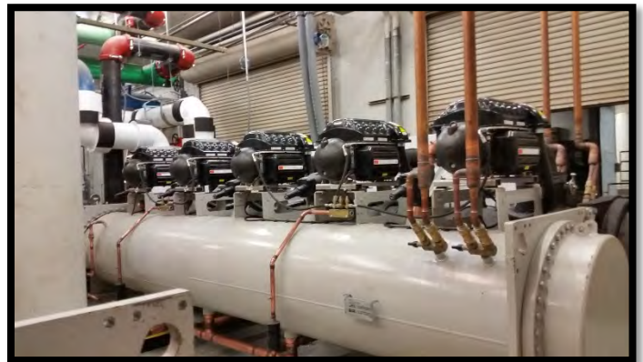
One of Two New 850 Ton Chillers
